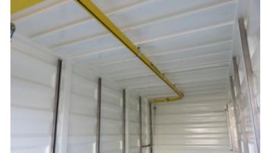
Internal monorail and unistrut
