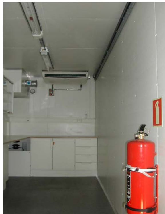
AC supply unit mounted under the ceiling
