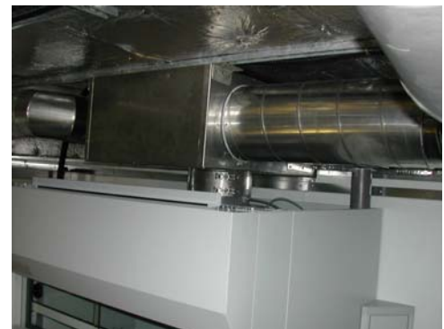
Extract ductwork from the fume cabinet
